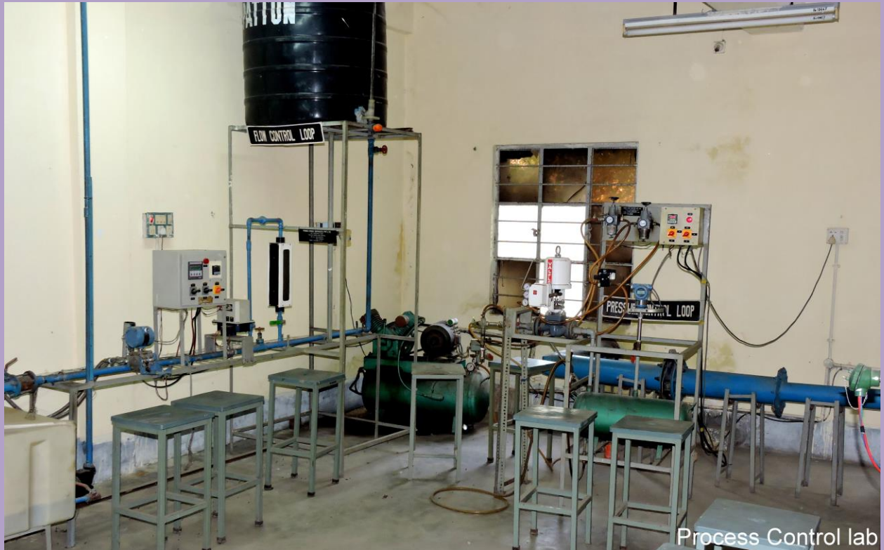
Process Control Lab
